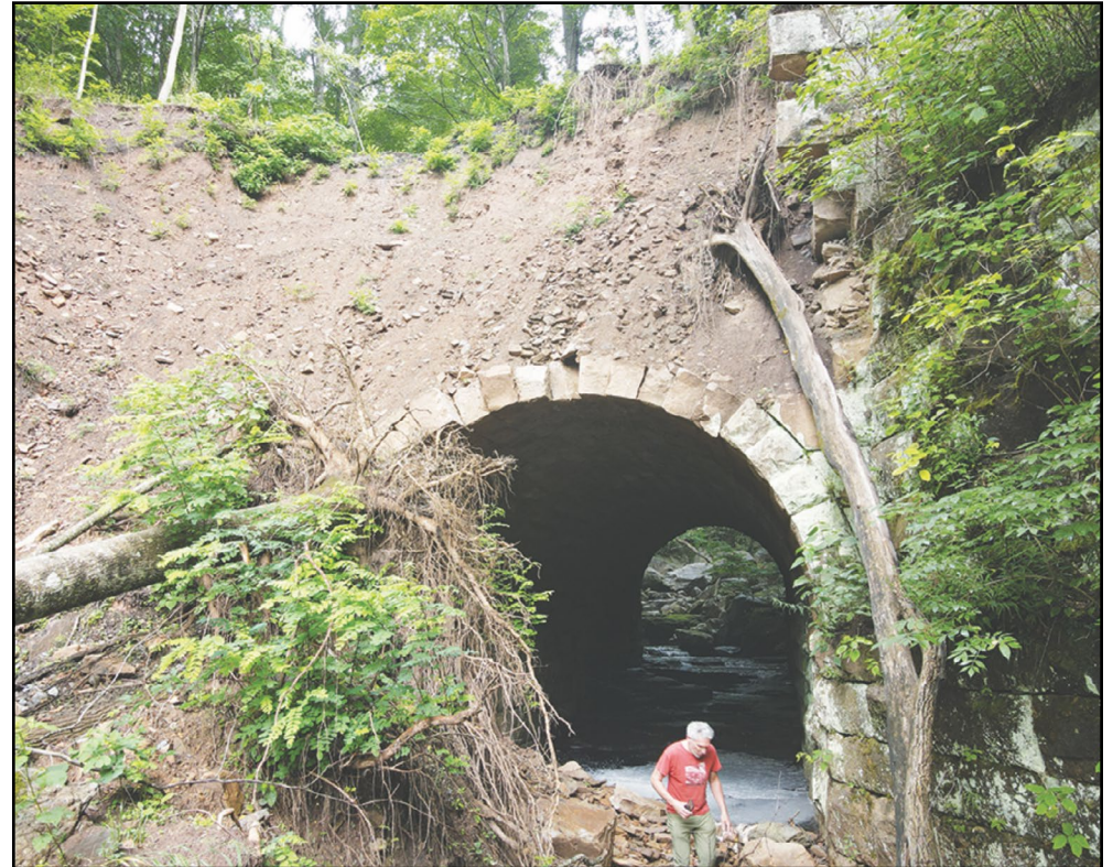
Severe damage caused by the Big Run Culvert along the Blackwater Canyon Trail. (Photo courtesy Stephen Strother.)
