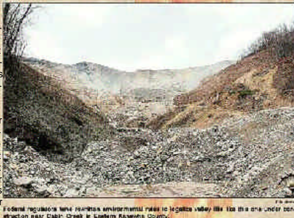
Federal regulations have rewritten environmental rules to legalize valley fills like this one under construction near Cabin Creek in Eastern Rappahannock County.
