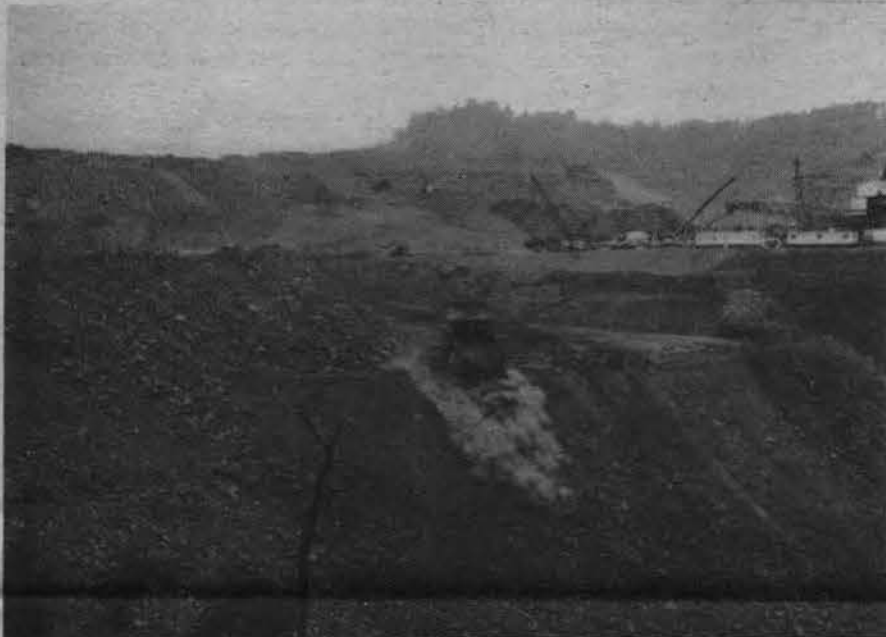
Looking across a valley fill in Southern WV during construction of first few 'lifts'.
