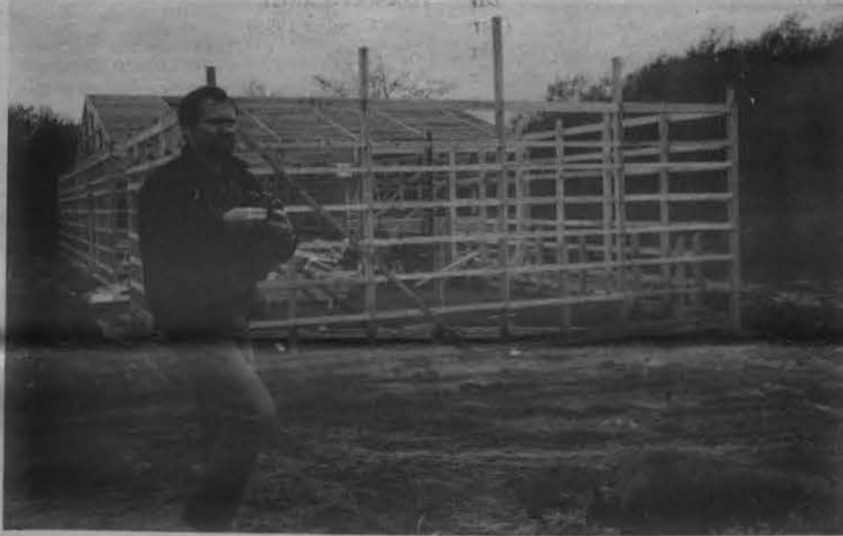
Richard diPretoro (new WVHC Administrative Assistant) at site of lime drum structure being constructed on the Blackwater River above Beaver Creek
