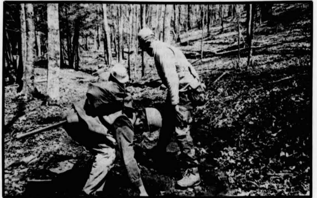
Conservancy members help construct a water bar on a trail in the Laurel Fork Wilderness during the Spring Review weekend. Their efforts were part of the Sierra Club's cooperative trail recovery project in the Monongahela National Forest.
